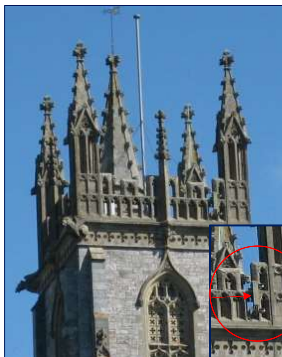
St Michael, Heavitree (The antennas are mounted to the face of the parapet)
